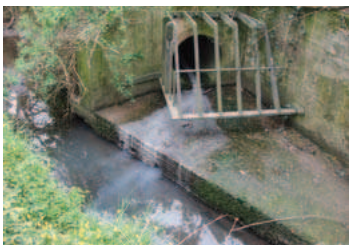
For decades, during dry spells, this white substance has been oozing out into Arrove Brook from two freshwater land drains along the Lane. One drain is 15 yards from Glenwood Drive bridge towards Arrove Brook Road and the other is 30 yards in the other direction. However, little shoals of Jack Sharps still survive in the water close by.
