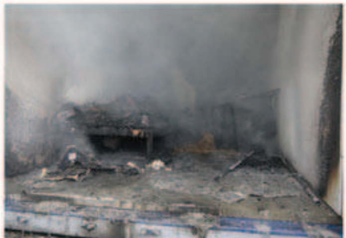
Damage of Fire after being extinguished by firefighters around 4 minutes after igniting. No mist system installed.
